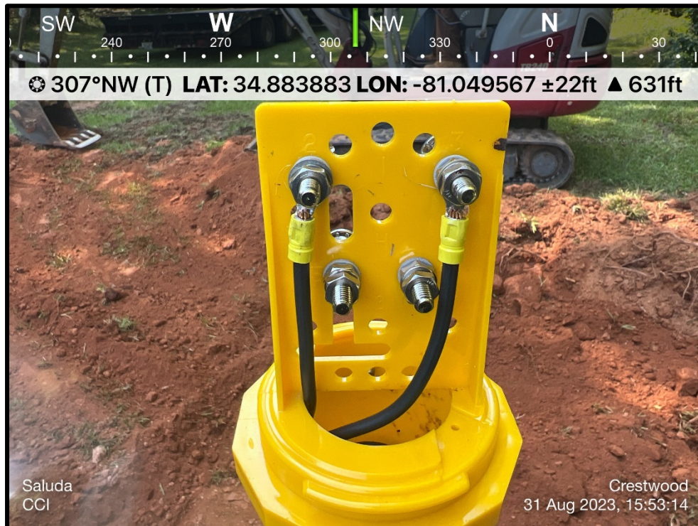
S-3: Pipeline test leads.
