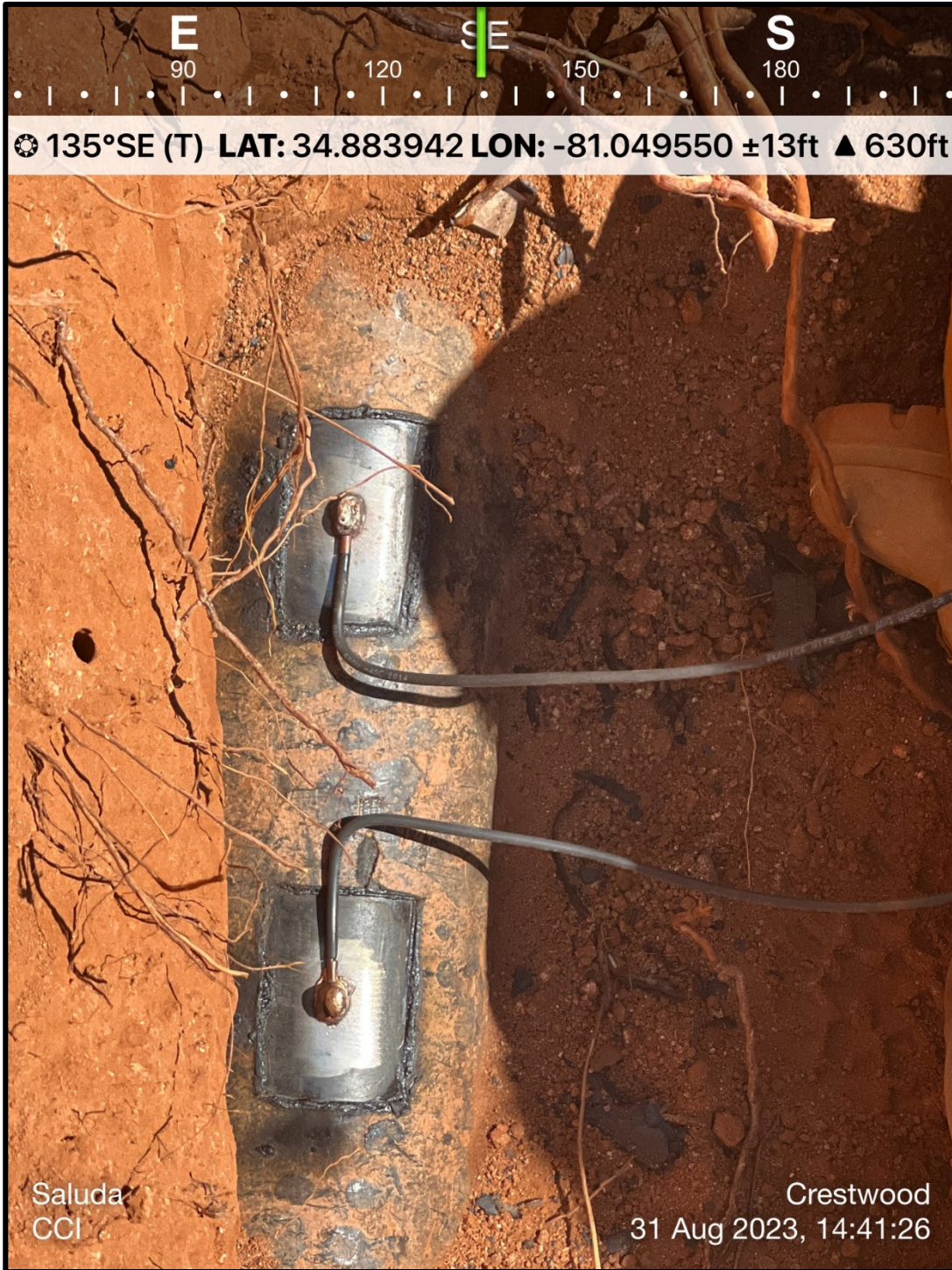
S-1: No. 10 wires attached to pipe.
