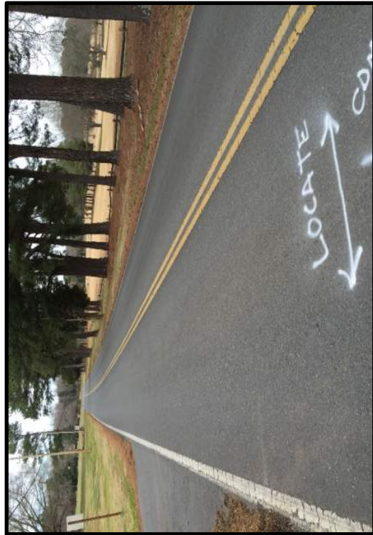
Looking north from near station 16+70 Harper Gault Road toward the intersection of SC72 and Harper Gault Road
