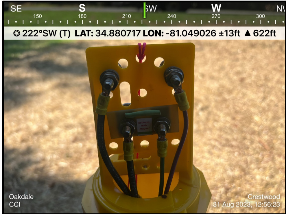
O-3: Pipeline wires (left) connected to one of two coupon wires (right), with a magnetically activated switch.
